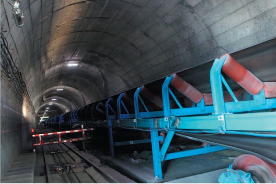
Fig. 10. The conveyer belt. The space between brackets is about 3 m.
